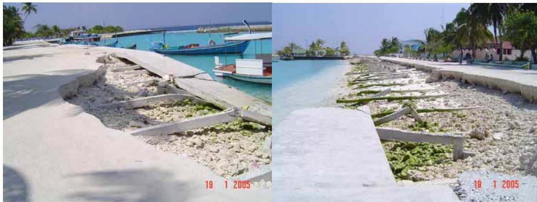
Plate 10. Tsunami damage to harbours and keywalls
