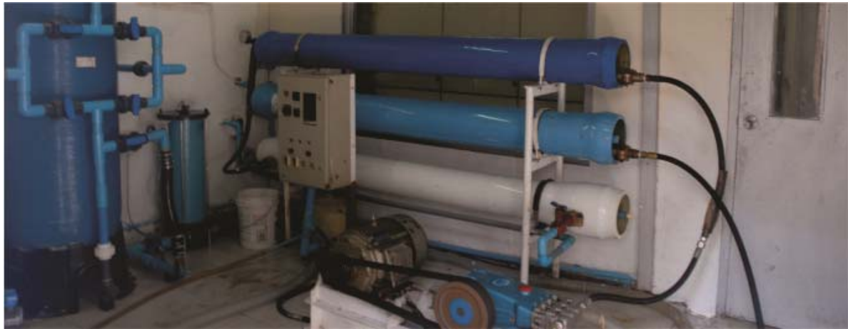
Figure 2: The RO plant at Kandholhudhoo
