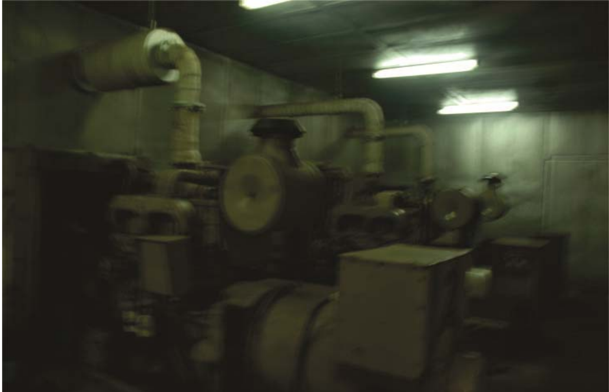
Figure 10: Diesel Generators at Kandholhudhoo
