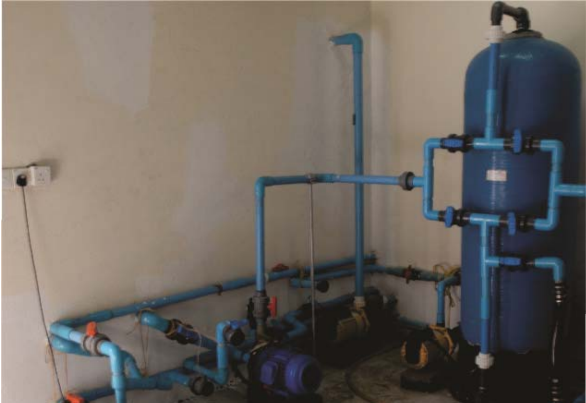
Figure 3: one set of sand filters and check filters at RO plant house
