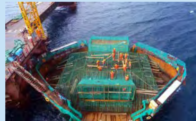
On the left is a photo showing the reinforcement of the pile cap and the start (skewback) of the arch legs.
