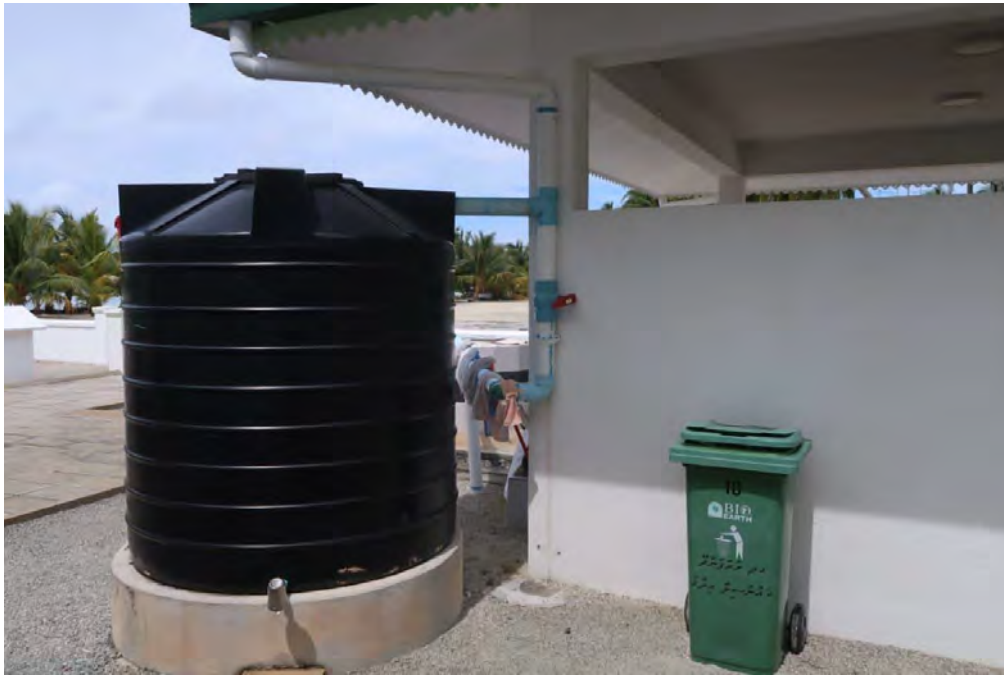
Figure 1.3: A simple Rainwater Harvesting setup in a mosque in GDh. Rathafandhoo (The most common method of Rainwater Harvesting system in islands) (Source: Authors)
