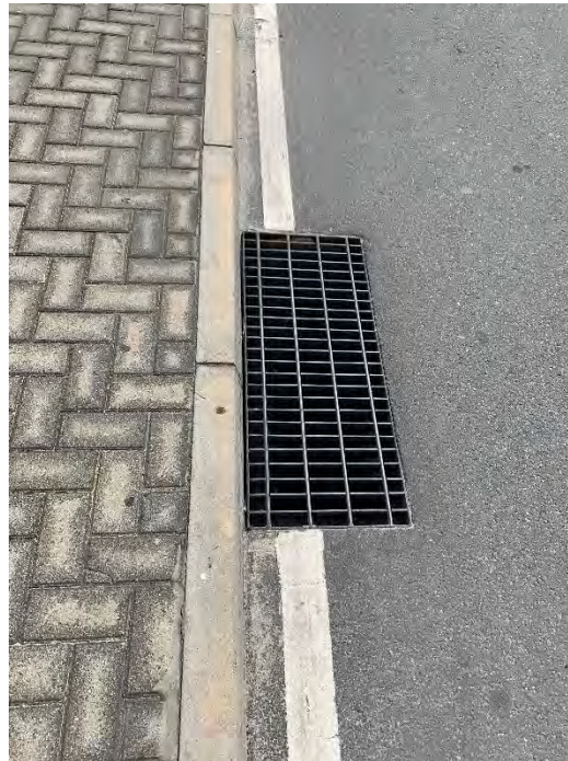
Figure 2.5: Grating of a road drain inlet installed in the ring road of the capital city Male' (Source: Authors)
