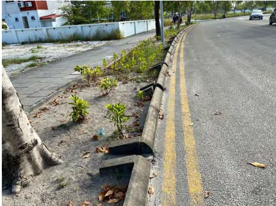
Figure 2.12: In almost every street in Hulhumale', stormwater is managed entirely by infiltration drainage facilities without using a piped drainage system. (Source: Authors)
