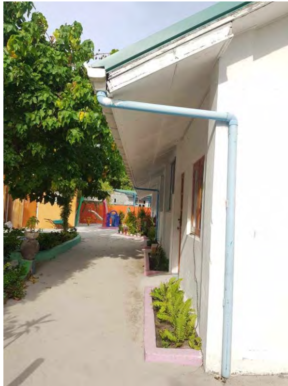
Figure 8: A downpipe connected to the roof gutter has been left to discharge rainwater directly to the ground surface (a common practice in the islands) (Source: Authors)
