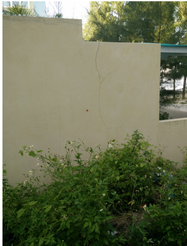
Southern boundary wall Cracking
