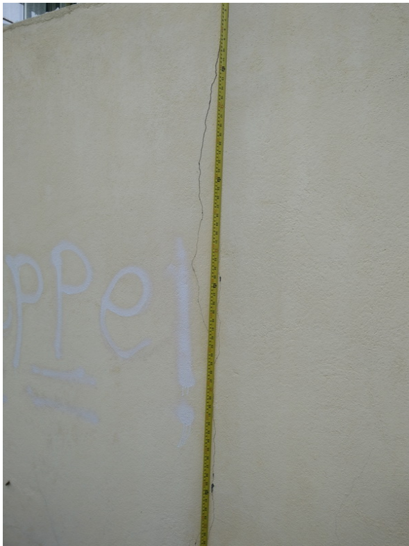
Southern boundary wall Cracking
