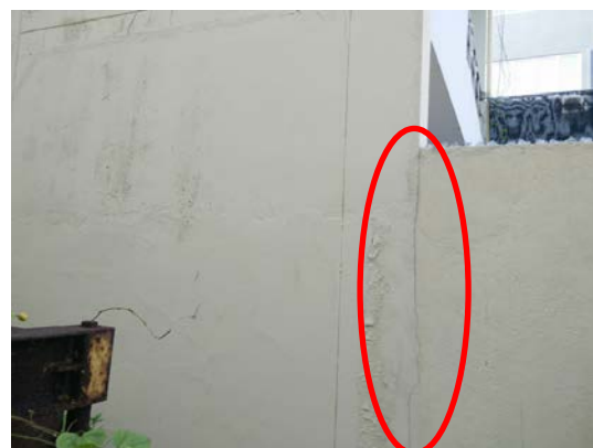
Southern boundary wall Cracking
