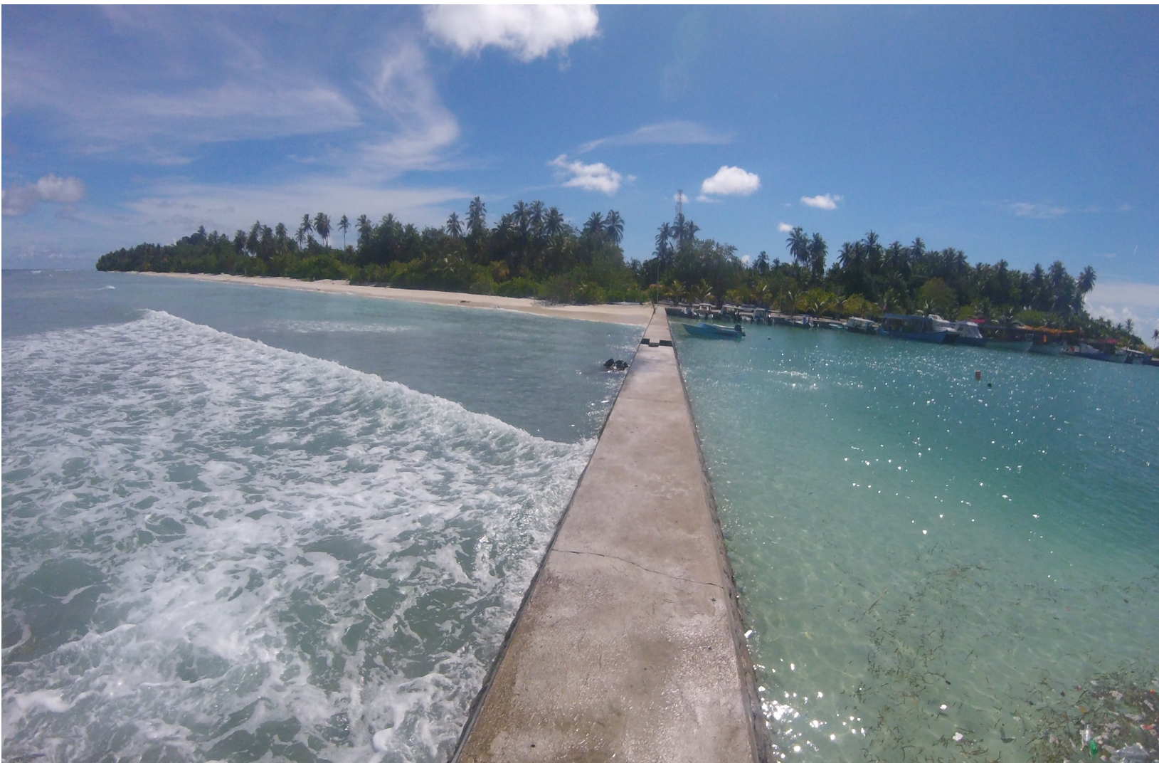
Figure 5.9: Photo showing the harbour wall. To the right of the wall is the harbour. To the left of the wall is the location of sites 1 – 22 stretching into the distance.
