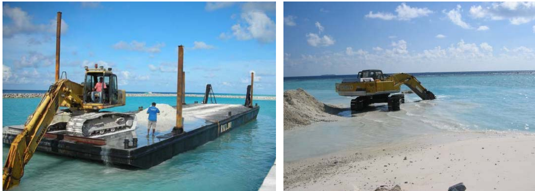
Figure 3: During the excavations works the dredger may be loaded onto a shallow draft barge (for deep harbors) or excavator sits on the site itself and works from the far end move to beach.
