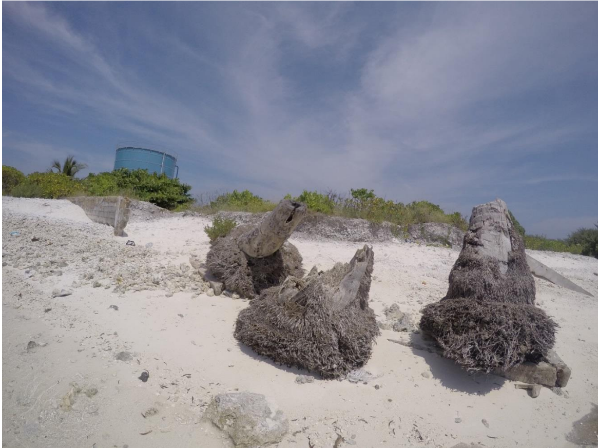
Figure 16: erosion at the corner of the desalination plant premise walls
