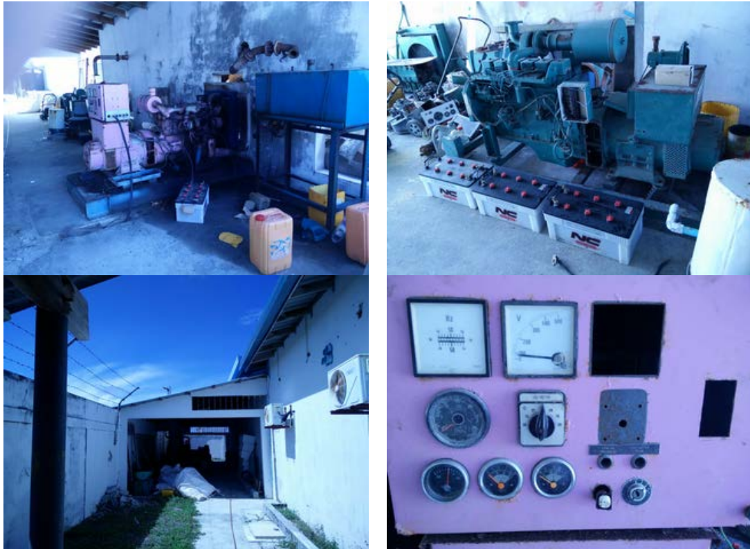
Figure 7: Existing generator sets top, powerhouse (bottom left) Penal board (bottom right)
