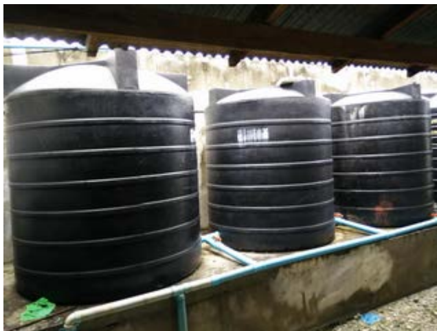
Figure 8: Existing rain water harvesting and storage tanks
