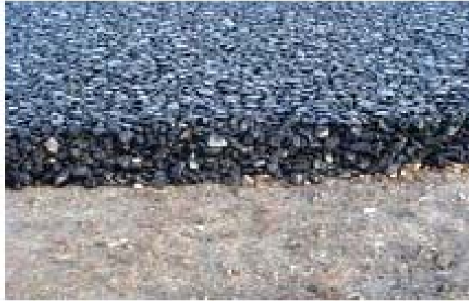
Figure 9: Rock aggregate base layers (bottom) with porous asphalt layer on top required for the air-field. Image extracted from Naeem et. al 2008.
