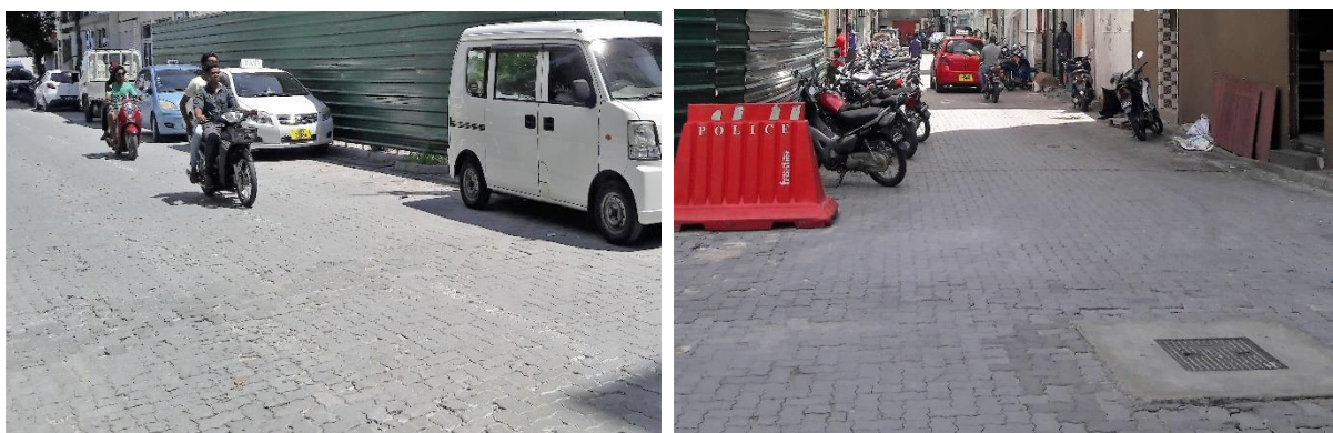
Figure 33: Condition of Boduthakurufaanu Magu (left) and Burevi Magu (right).
