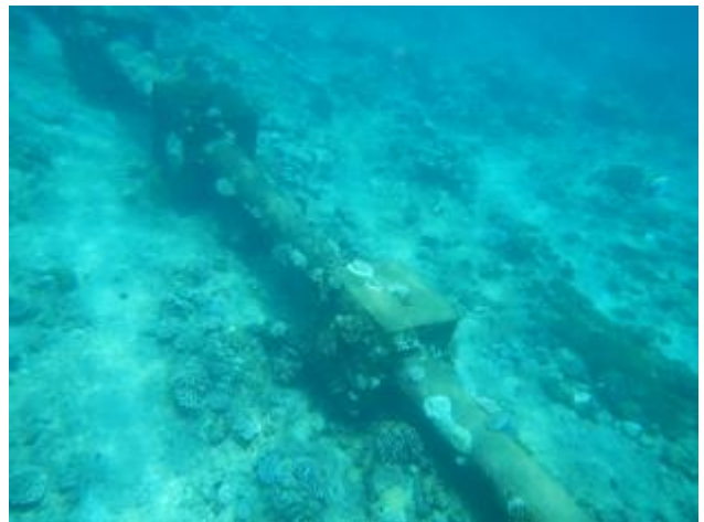
Figure 4.24: Sewage outfall pipe anchored near the cable deployment site
