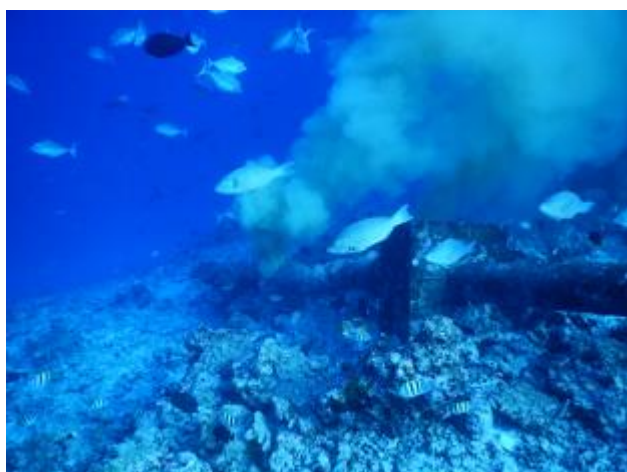
Figure 4.42: Sewage Outfall pipe anchored to the reef slope
