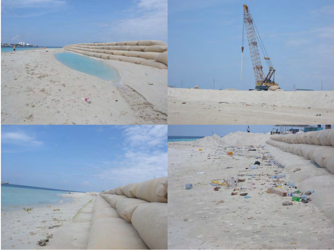
Figure 4.13 Coastal protection activities being carried out on the south western and western side.
