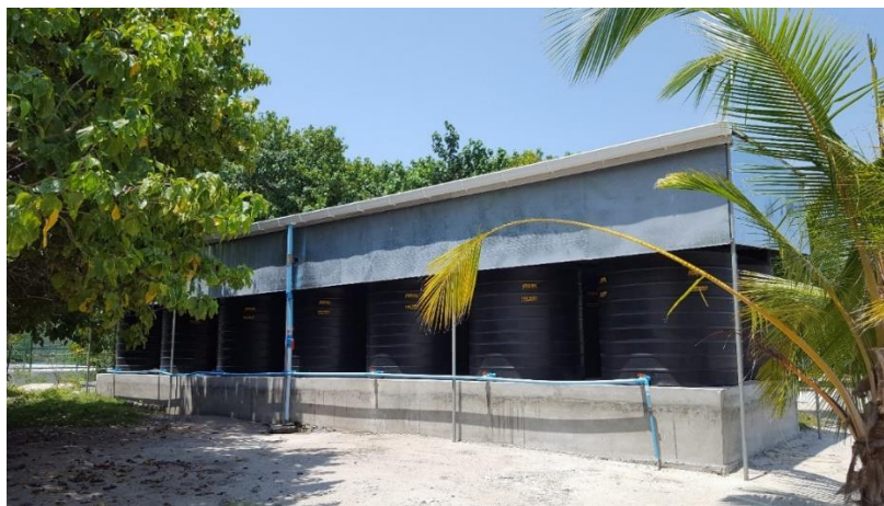
Figure 22: Public rainwater harvesting and distribution systems present at Sh.Foakaidhoo
