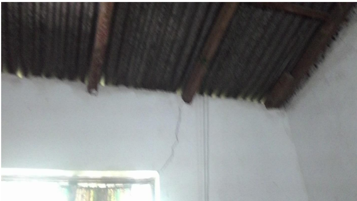
Figure 24: crack lines in house
