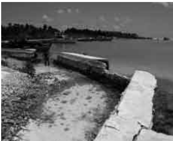
Partially collapsed seawall at Faafu Nilandhoo
