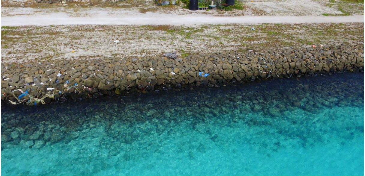
Figure 94: Rock revetment used to protect coastline at Gulhifalhu
