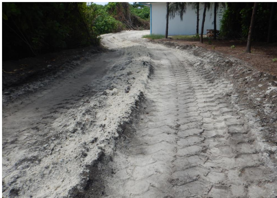
Figure 97: Damage caused to sand-surfaced road in an island by heavy vehicles
