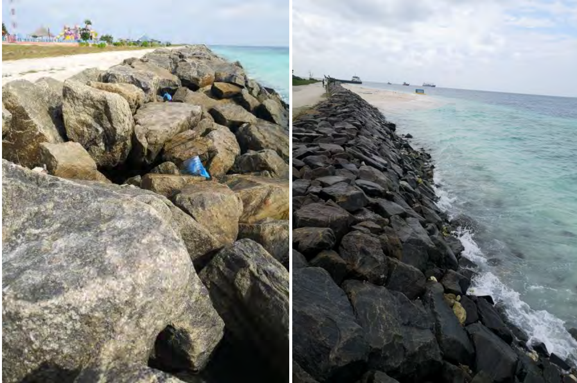
Figure 21 Revetment structure condition in B. Eydhafushi
