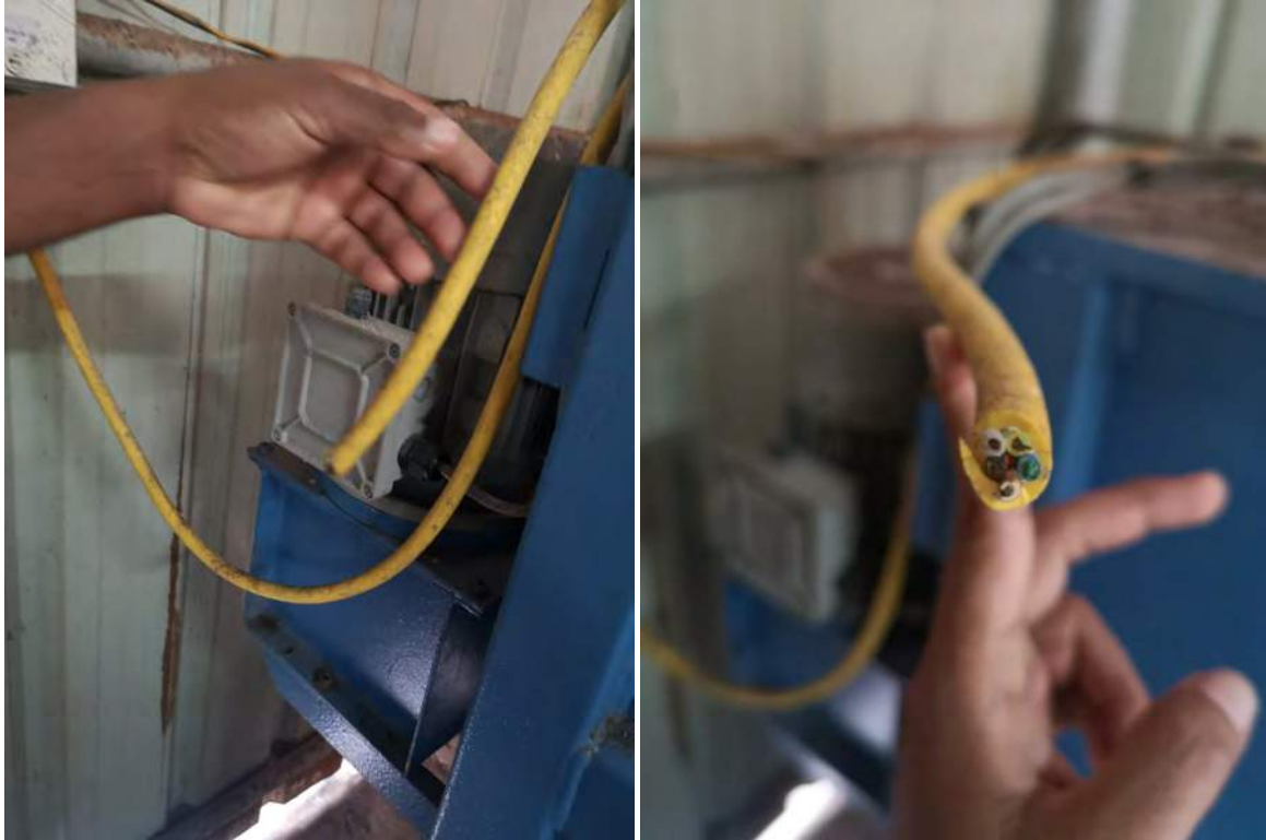
Figure 15 Power cables to all the machinery at the IWMC had been damaged
