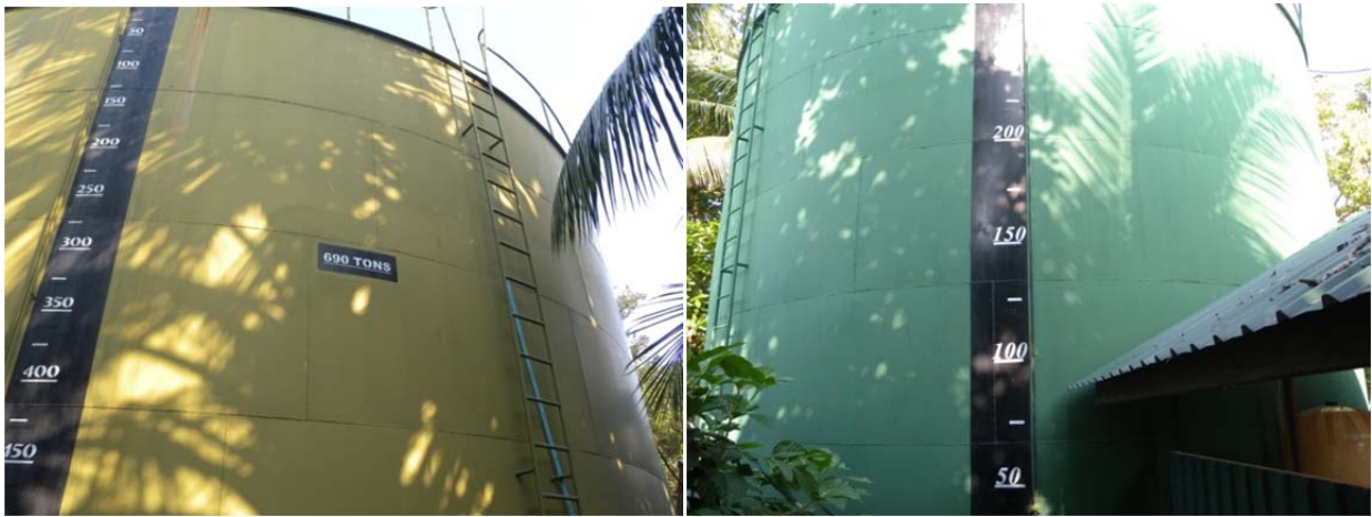
FIGURE 4-5 STORAGE TANKS OF DESALINATED PLANTS
