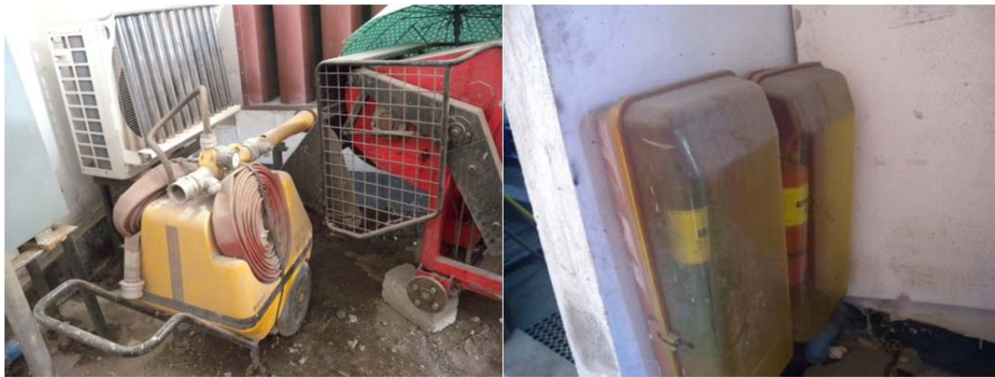
FIGURE 4-6 HI COMBAT AF 120 MOBILE FOAM UNIT (LEFT) AND FIRE EXTINGUISHERS INSTALLED INSIDE DESALINATION PLANT HOUSE (RIGHT)
