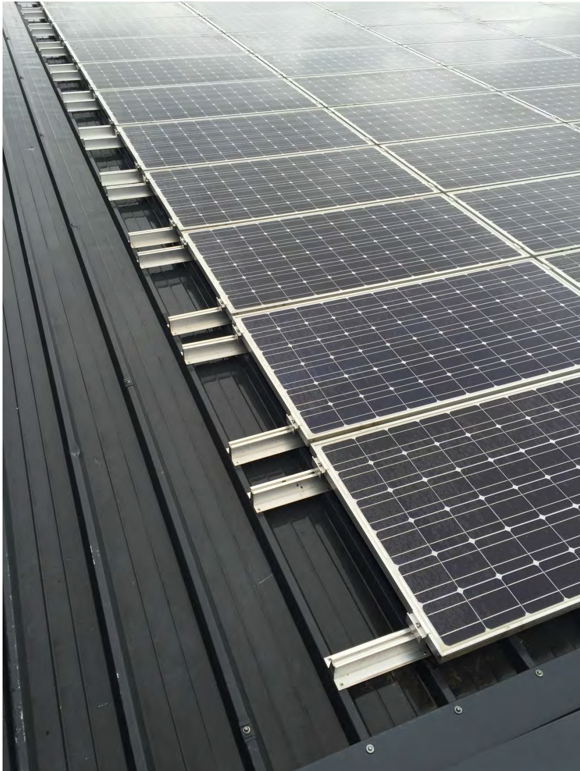
Figure 8: Substructure crossbar with PV modules
