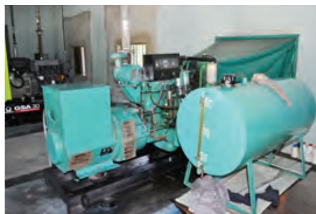
A diesel generator installed at a powerhouse
