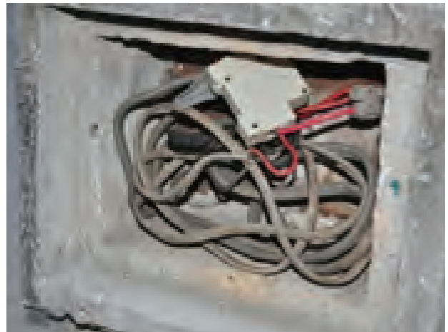
Distribution box at an island
