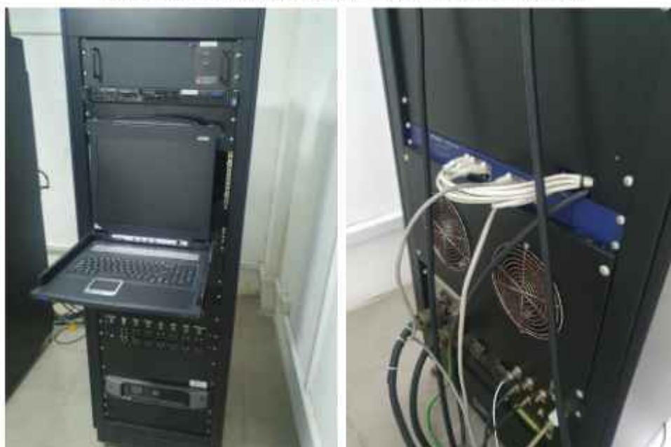
Figure 18: Current status of the Malé radar server rack
