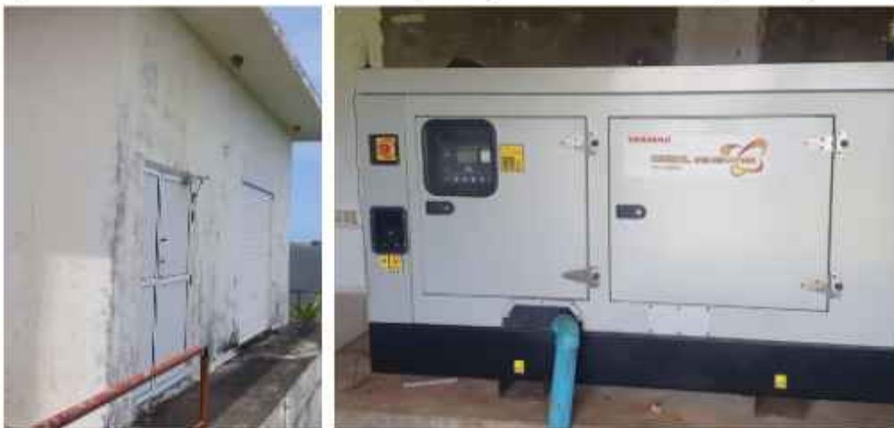
Figure 16: Current status of the Malé power generator room and power generator
