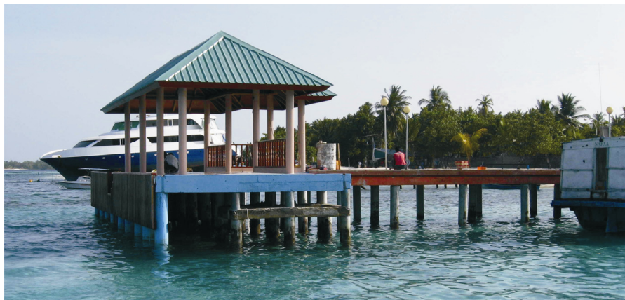
Figure 2-3: Jetty located on western side of the island accessing to the natural harbour.
