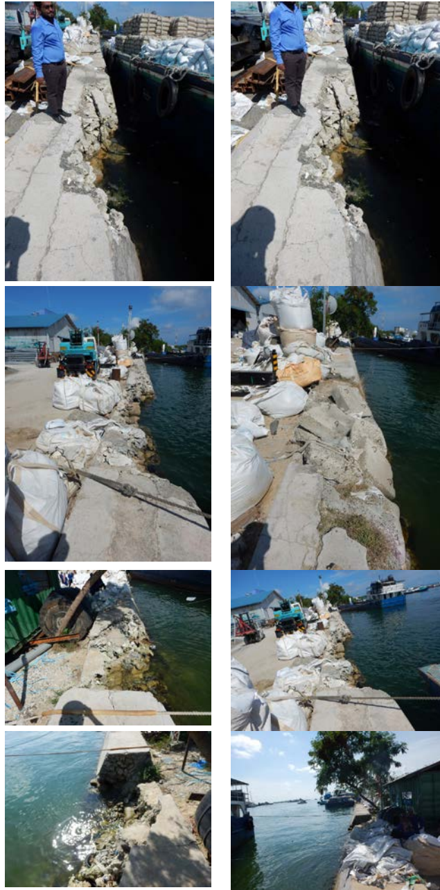
Figure 14: Existing quay wall broken into pieces unsafe to use, totally destroyed
