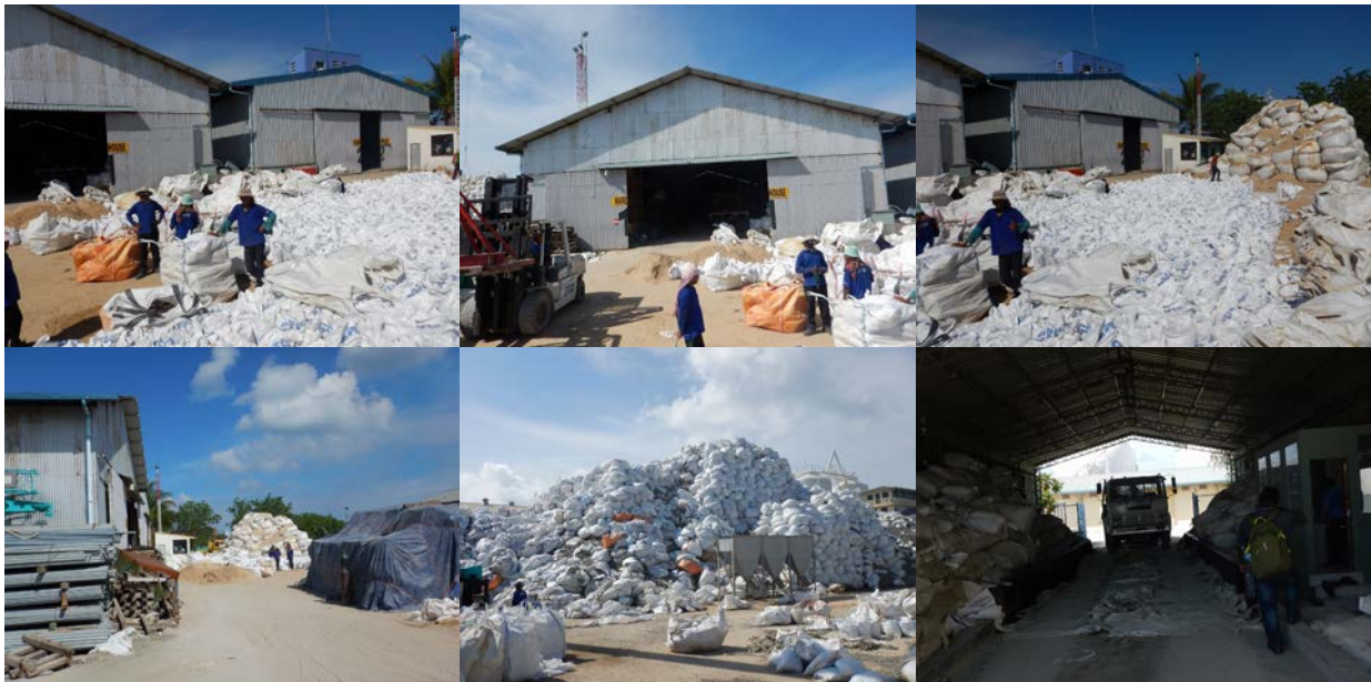
Figure 13: Nature of heavy operation in STO Plot 2 loading and unloading sea and land transportation and storage of construction material.
