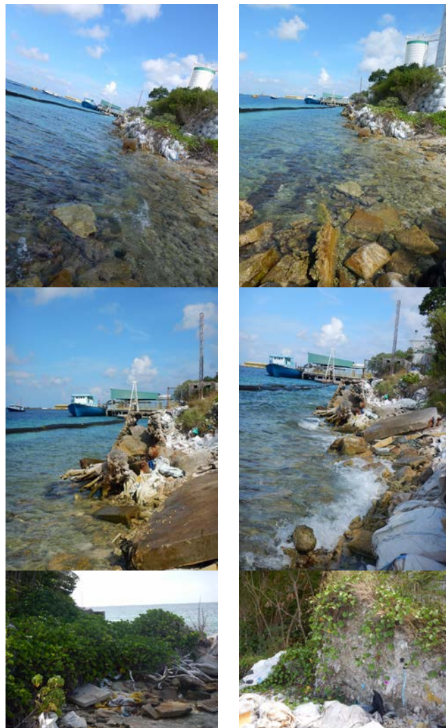
Figure 16: Damages seawall STO plot 111
