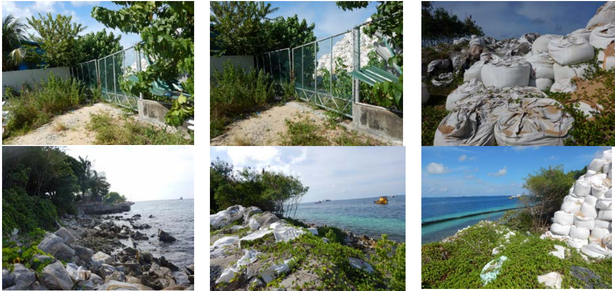
Figure 15: land and seaward boundary of the STO plot 111, showing damaged seawall and subsequent washing away of stored construction material
