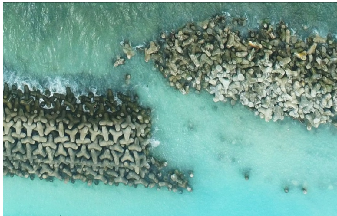
The tetrapod breakwater was being moved seawards with a large percentage breakage of the tetrapods.
