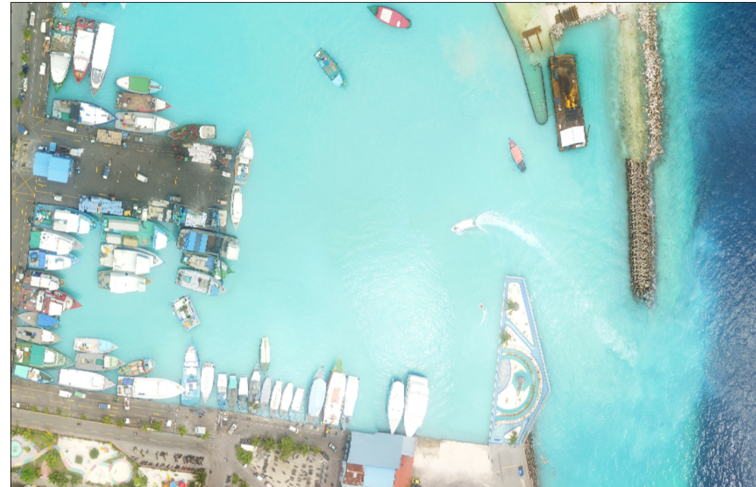
Sheet pile wall has been completed at the T Jetty area. The dredging works caused sedimentation inside the harbour area, however, the movement outside an onto the reef is slow and at lower levels.
