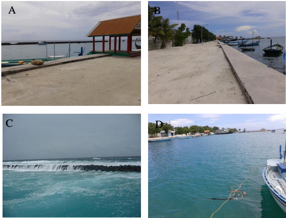
Figure 1: Condition of the existing harbour of Inguraidhoo Island compared during different weathers (A) Western side of the harbour damaged (B) Front side of the harbour as seen during calm conditions (C) submerged breakwater and overtopping waves during rough weather (D) Vessels moored in the harbour during a calm day
